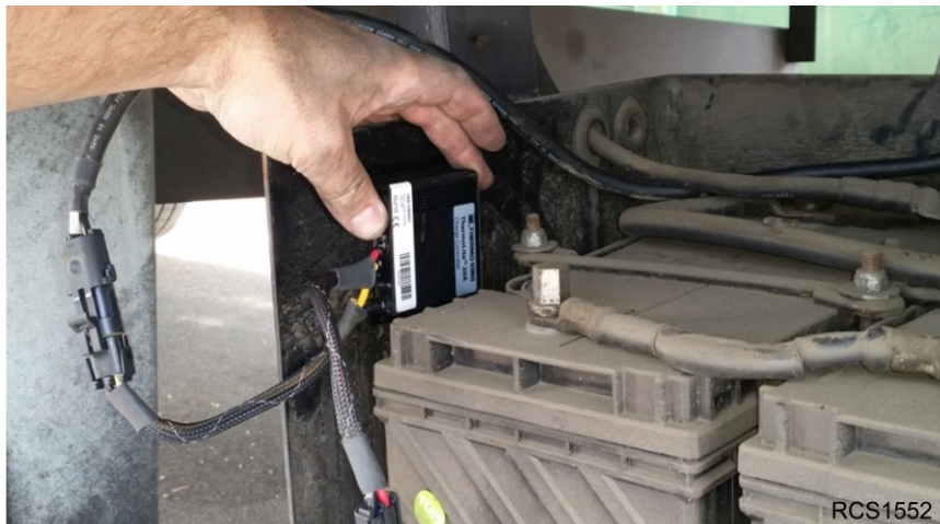
Figure 12. Secure Charge Controller near batteries.
