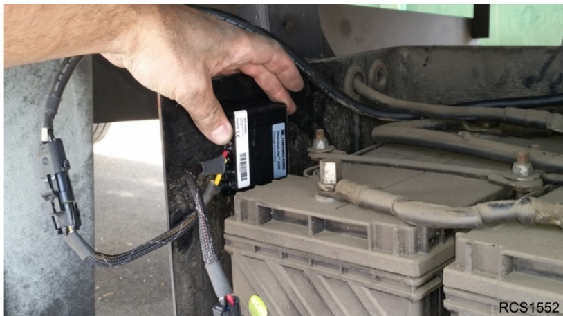
Figure 11. Secure Charge Controller near batteries
